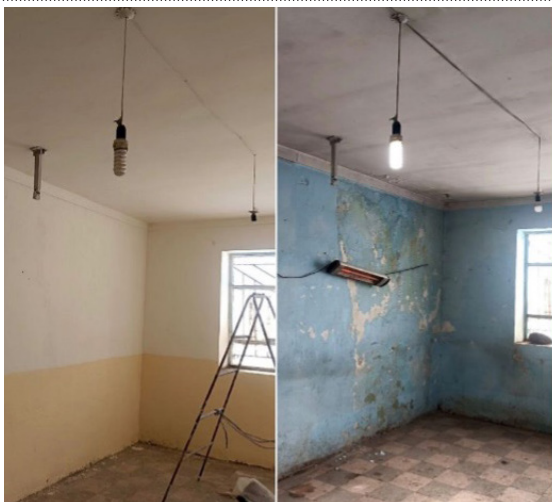
Photos: Mitra Ghaffarian (Khoy, Dec 2023)- Karkoush village Rehabilitation of damaged schools in earthquake
