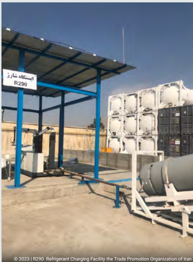
© 2023 | R290 Refrigerant Charging Facility the Trade Promotion Organization of Iran
